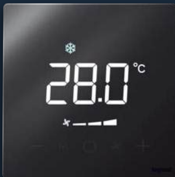
Room temperature control unit
